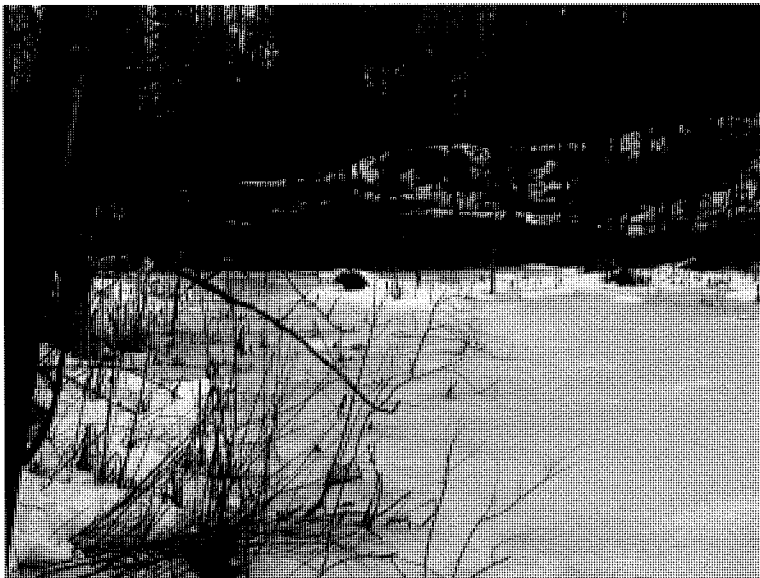
Photo 1. Brewster – Bridge (Brew 2) covered in snow and ice. Photo was taken during the March 30, 2009 survey.
