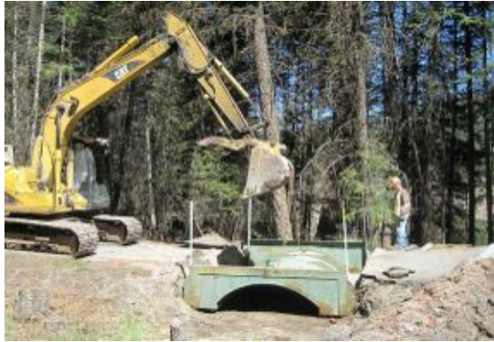
Installation of an underpass for Western Toad roadkill mitigation across BC Parks road, May 2013.
