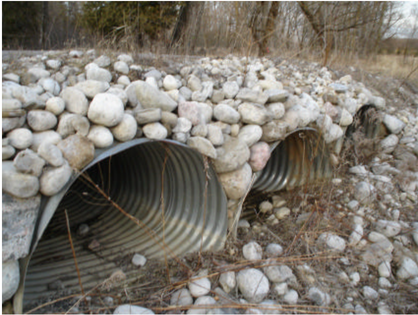
Figure 4: RIM Park: April 5, 2005. Culverts built for herpetofauna and water movement (Photo taken by author).
