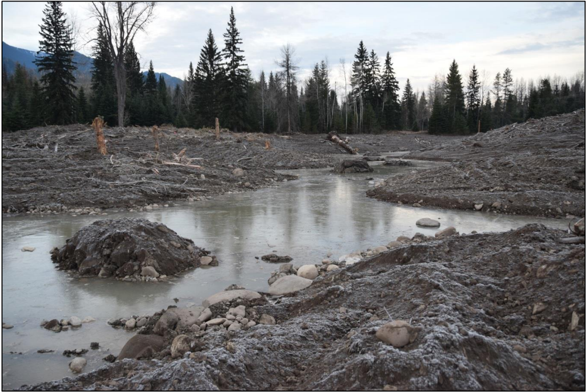
Figure 6. Completed wetland restoration of perennial wetlands PRL#1 and PRL#2 on October 31, 2017, Hosmer BC.
